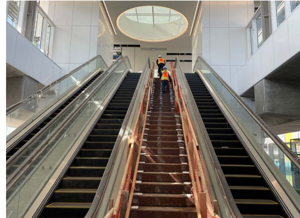
Escalators at ITFW Station
