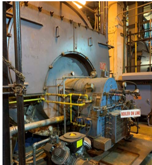
Example of existing boilers at Chelsea Houses
