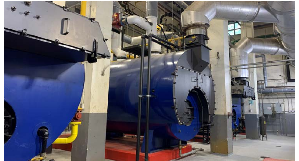
Example of upgraded boilers at Baychester Houses
