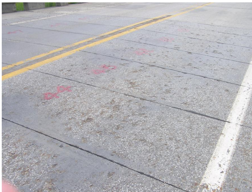
Figure 24. Deterioration of Eastbound Lane Slabs
