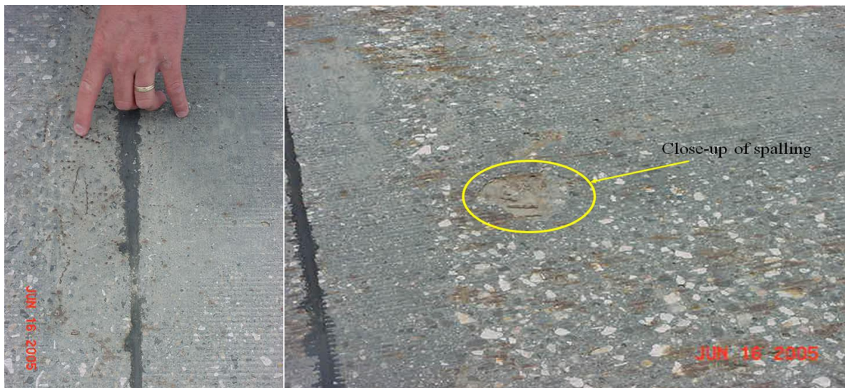
Figure 20. Close-up of exposed steel fibers and spalls
