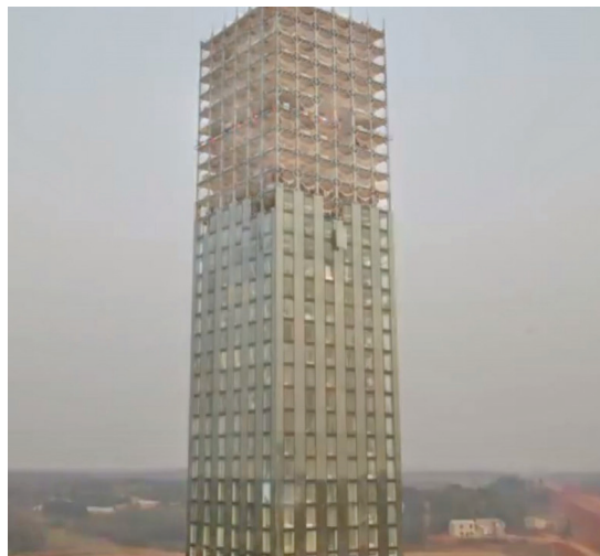
GOING UP A 30-story hotel in China, completed by BROAD Sustainable Buildings in only 15 days, is shown in a time-lapse video at hour 317 of the process.
