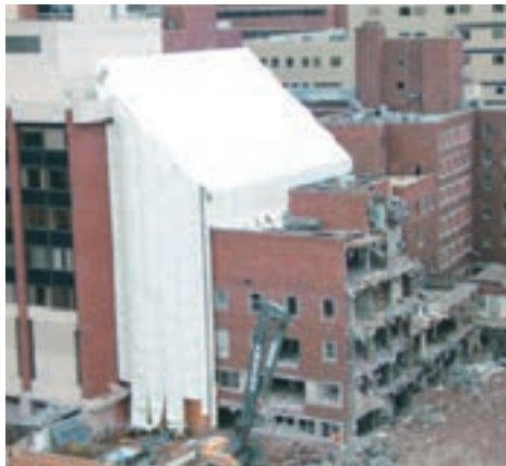
HAKI enclosure protected the Barnes Jewish Hospital in St. Louis, Mo., during winter demolition.
